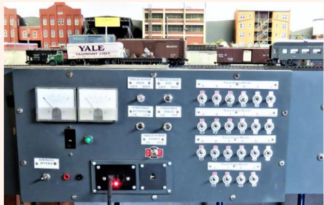
The layout was originally wired for DC Block operation. Using DPDT toggle switches the layout can change from DC operation to DCC operation. This allows the use of either old DC engines or newer DCC motive power. The rest of the layout wiring did not change.
