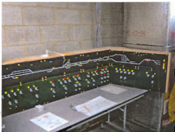
Steve Mallery's Dispatcher Panel
